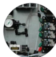
Pneumatic control systems
